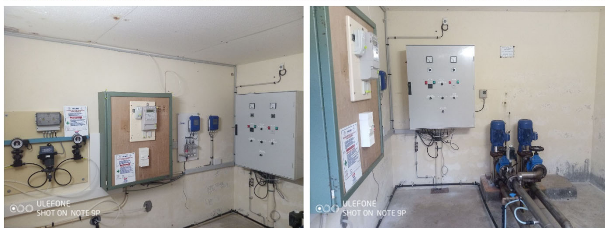
Figure 16 : station de pompage Rousson.
